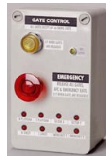
Electromagnetic Lock Control & Status Panel
